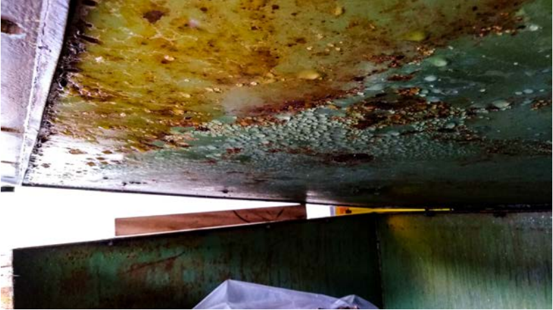
Figure 2 - Inside of the box that showed the highest moisture content. Note the water droplets formed by condensation in the underside of the box lid.
